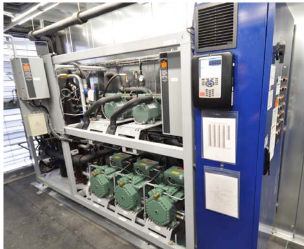
Figure 1 - Booster System Rack
