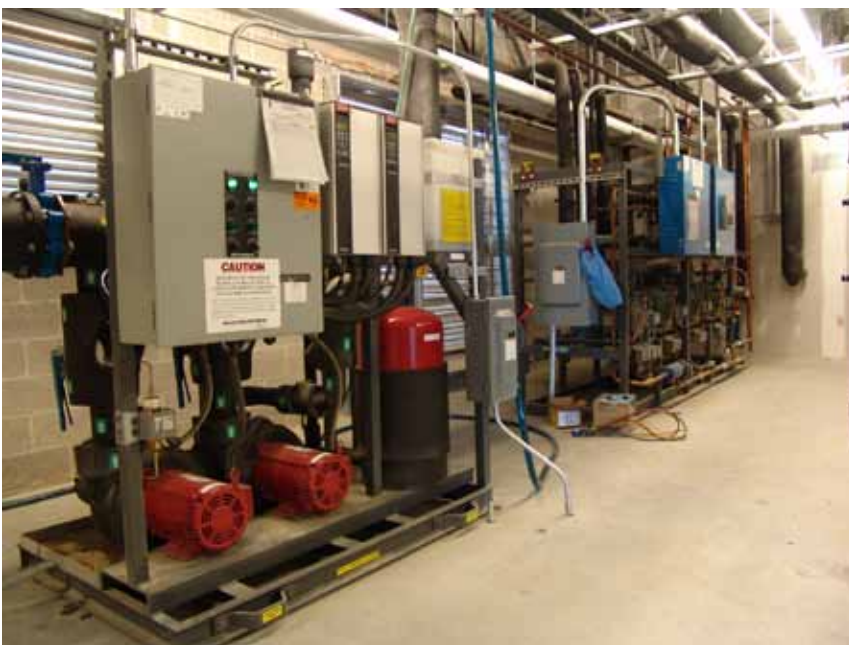
SNMT system equipped with variable-speed (VS) inverter-controlled pumps
