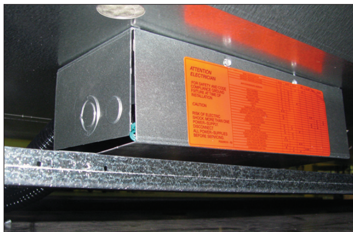
Fig. 14 Junction box beneath case
