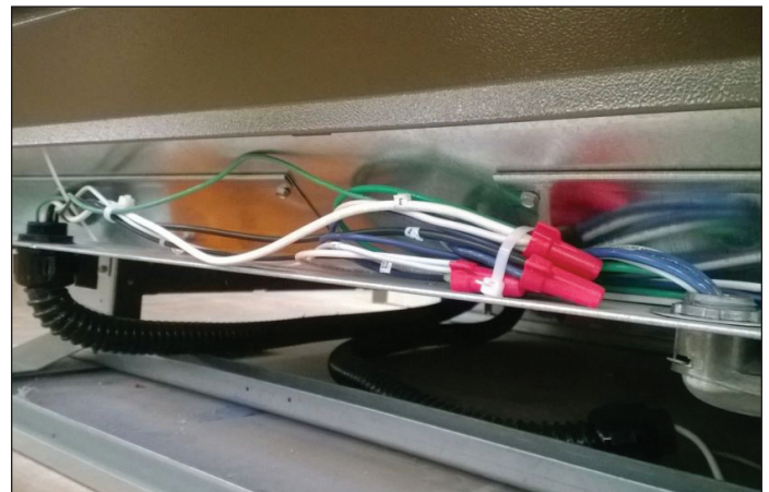
Fig. 7 Raceway electrical wiring
