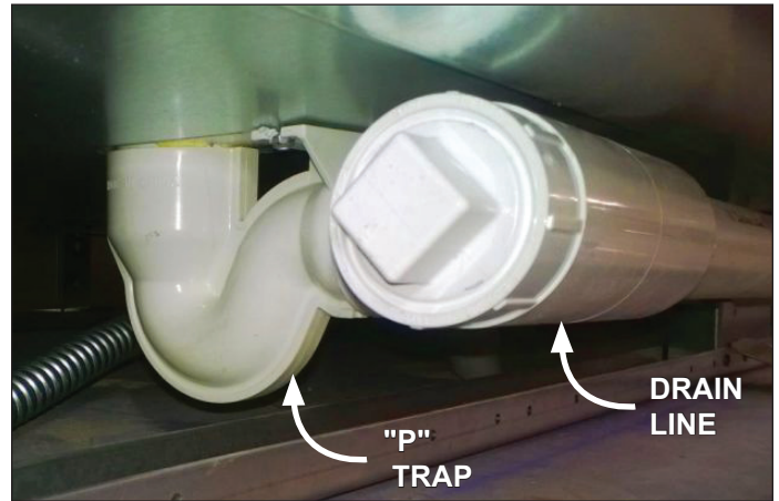
Fig. 6 “P” trap; drain line
