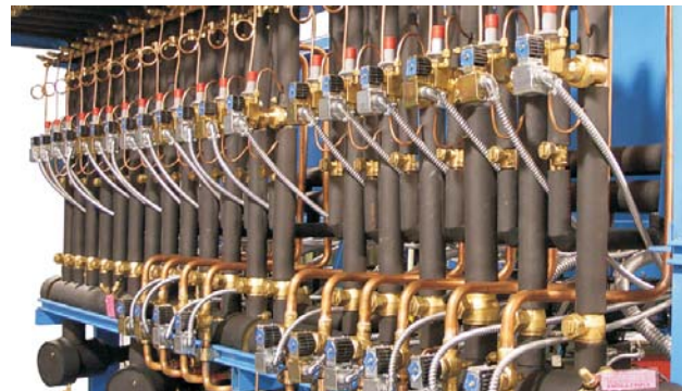
Manifold piping on HRP rack.
