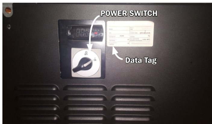
Fig. 7 Lower panel switch locations
