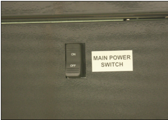
Fig. 11 Lower panel power switch
